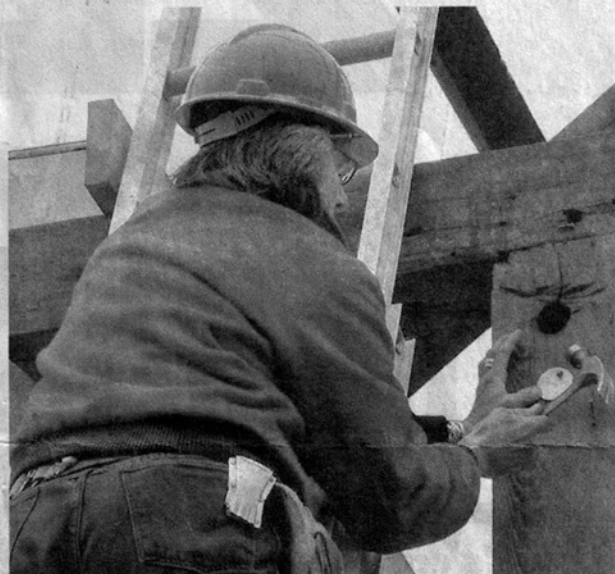
Ellen Gibson is a member of the Timber Framers Guild, which disassembled the barn and numbered about 600 pieces.
